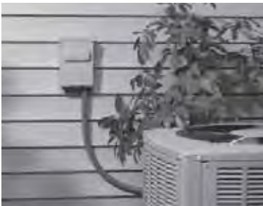
As an air conditioner disconnect
